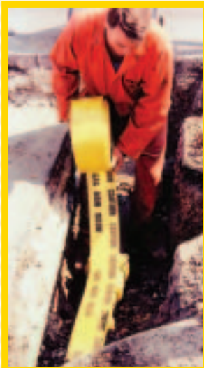
Gas pipe protection roll
